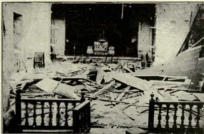
INTERIOR OF THE CHURCH OF GUBAT ONE DAY AFTER THE TYPHOON.
